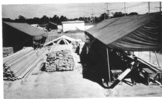
The field shop where rough lumber is cut to proper lengths and where such items as roof trusses are built.
