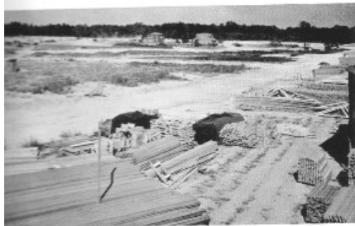
Construction site for 300 houses at Aero Acres. Materials in the foreground are piled behind the field shop, ready for distribution.
