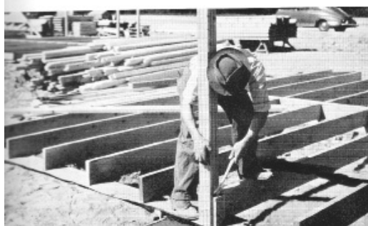
The first wood column is set in place against a floor joist. The columns are manufactured at a millwork plant and shipped to the building site.
