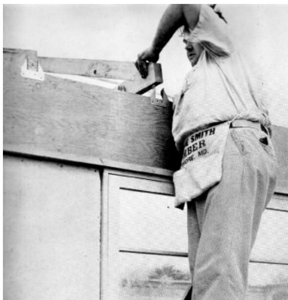
The end of a roof truss is being dropped into a hurricane clip. The clips are attached to the wall girders before the girders are delivered to the house site.
