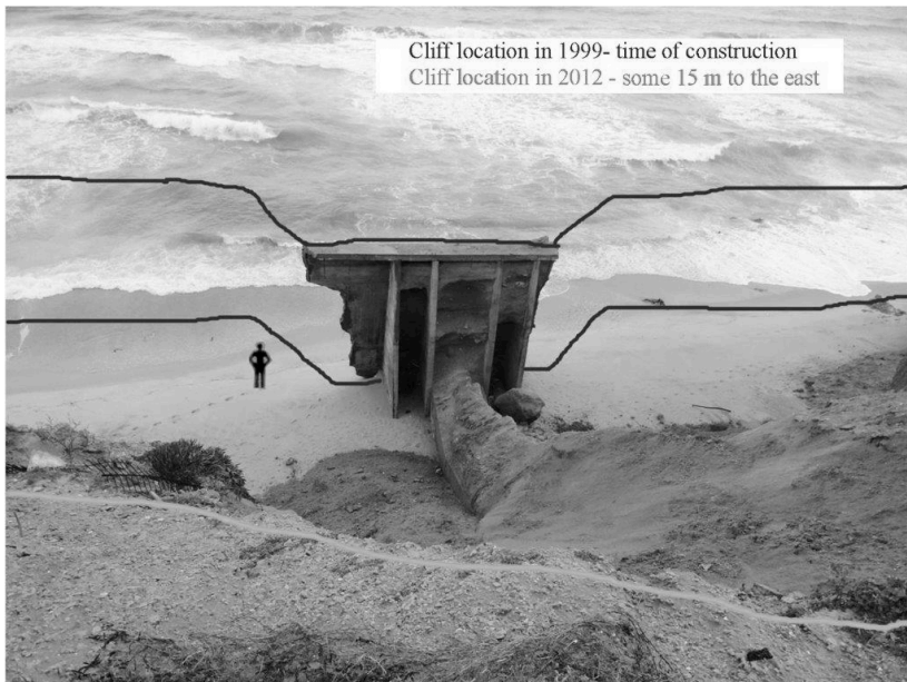
Fig. 12 - A sewer outlet in Ashkelon North, demonstrating the cliff retreat of more than 1 m yearly. The two upper lines depicts the location of the coastal cliff in 1999 and the lower line indicates the present cliff edge.
