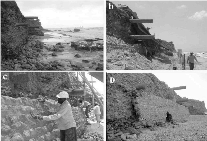
Fig. 14 - Ashkelon sea wall under reconstruction works: a) before works, b, C) a protective layer is being built on the wall face, D) the protective layer underwent erosion by the storm waves.
