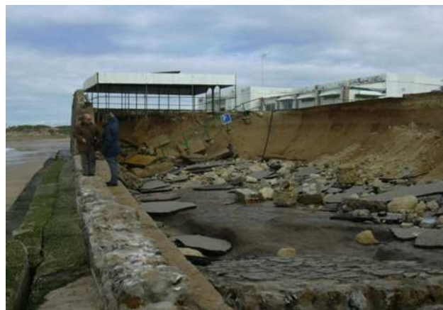
Fig. 5. Destruction of Punta Candor protruding paved area after the storm of December, 2004.
