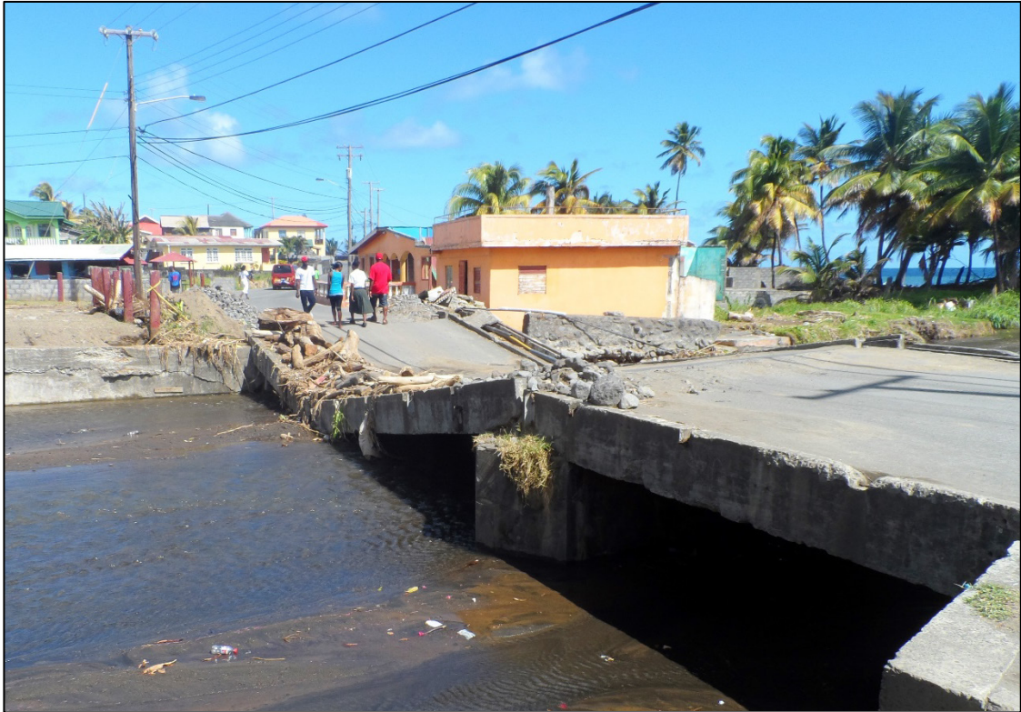
Plate 3.1. Photograph taken during fieldwork in January 2014 showing the damage to a bridge in the town of Georgetown on the windward coast. This bridge is part of the Windward Highway which is the main access road along the eastern coast of the island, from Kingstown to Fancy.
