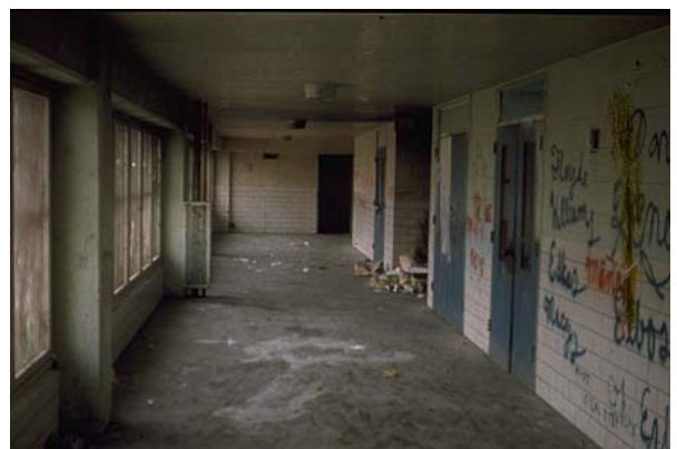
Figure 2: Vandalism in a communal corridor (Newman, 1996b).
