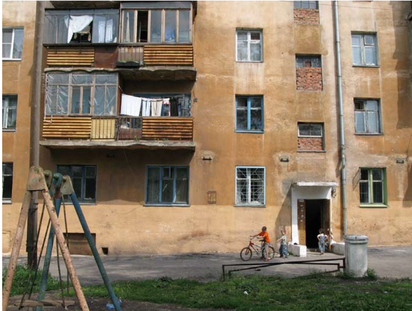
3.084 Front view of entrance and balcony of Socgorod super-blocks (1935) by Ernst May
