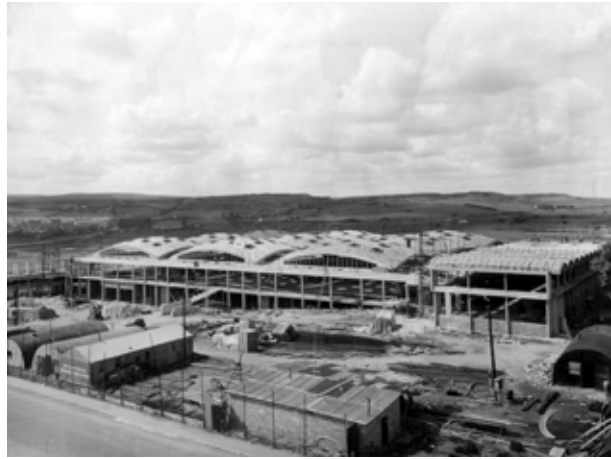
4.083 Factory for Brynmawr Rubber Company, Brynmawr, Gwent (1951) by Architects Co-Partnership, photo by Hylton Warner (RIBA18437)
