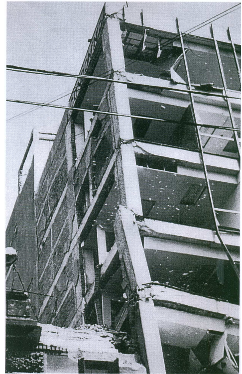
Figure 6.4: External BCJ failure in the 1985 Mexico earthquake. Source: Cheung, Pauly, Park [6-3] [1993]
