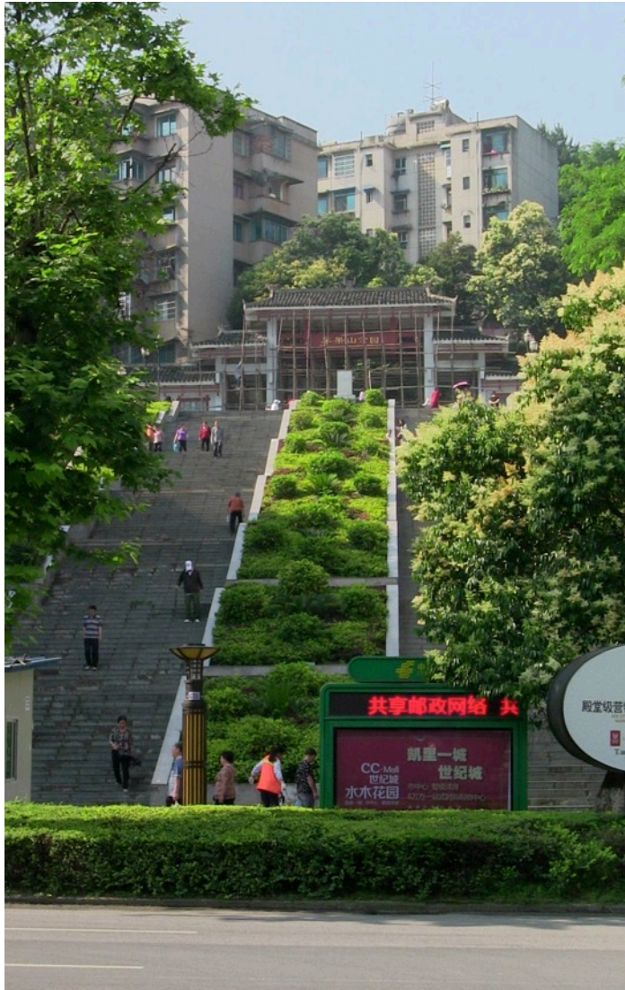
Figure 5.1: The main entrance to Apple Hill Park under repair (fieldwork photo 2013)
