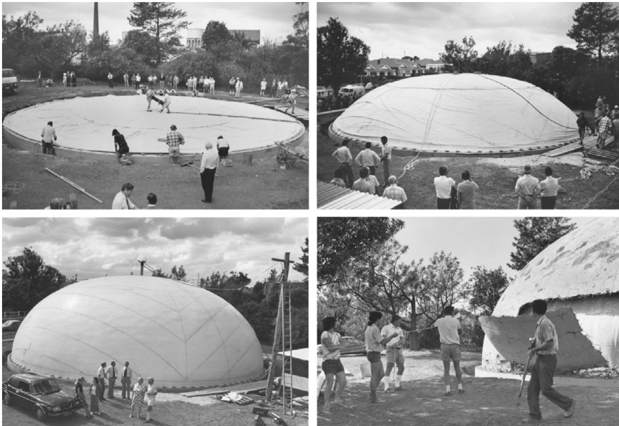
Figure 8. New South Wales, Australia. Architect, Dante Bini. Construction of Ashbury Public School administration building, 1973. Photographs: Max Dupain. Private archives of Dante Bini.
