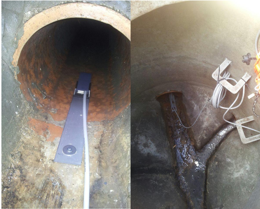
Figure 3.6: Installation of Stingray 2.0 UDFM equipment in surface water drainage manholes; (left) the installation of the sensor within the pipe upstream of the manhole; (right) the storage of cabling and data logging box.
