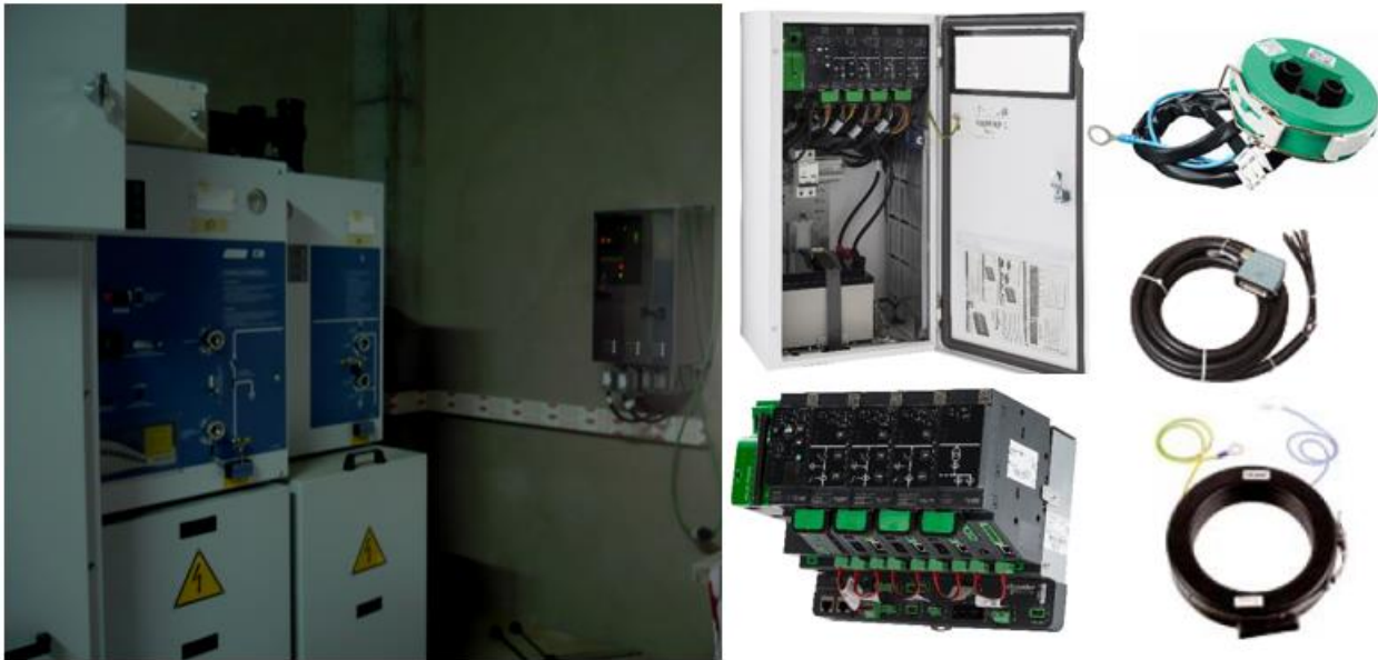
Figure 5.17 Example of telecontrol device in a MV-LV substation, courtesy of Schneider Electric
