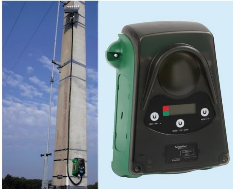
Figure 5.15 Pole mounted FPI with solar panel, courtesy of Schneider Electric
