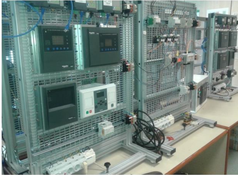
Figure 7.10 Interoperability between devices, courtesy of Schneider Electric
