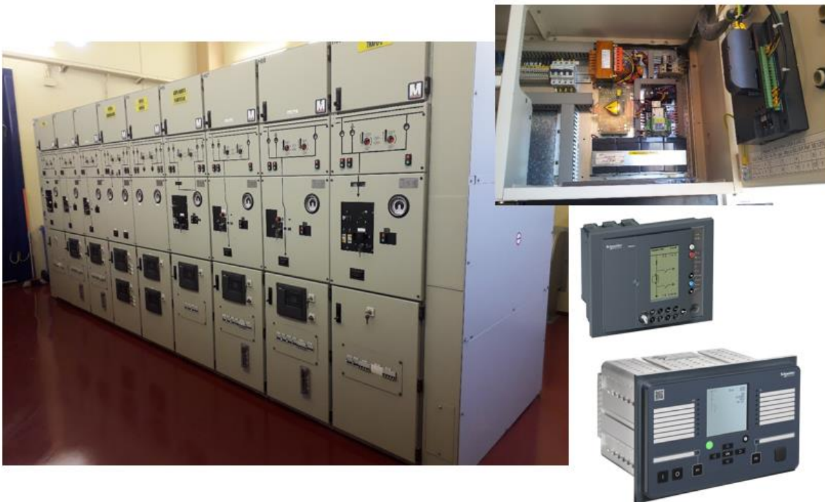
Figure 5.11 AEDs devices in some substation outgoings, courtesy of Schneider Electric
