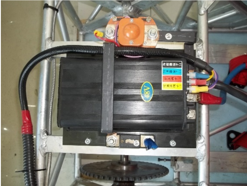
Fig. 3 The electric engine controller
