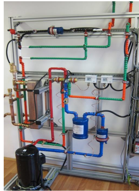
Fig. 2. Compressor based heat pump system
