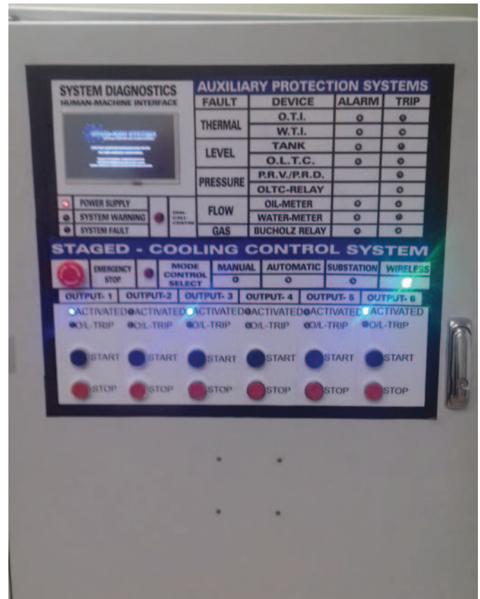
Figure 7: ACM system's user interface with cooling control panel
