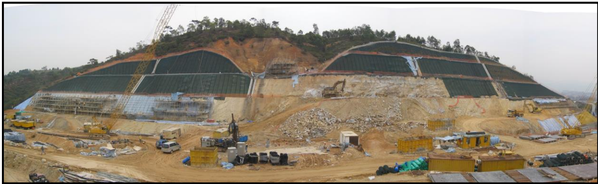
Plate 6 - General view of 40m high cut slope at northern end of Deep Bay Link during soil nail installation (March 2005)
