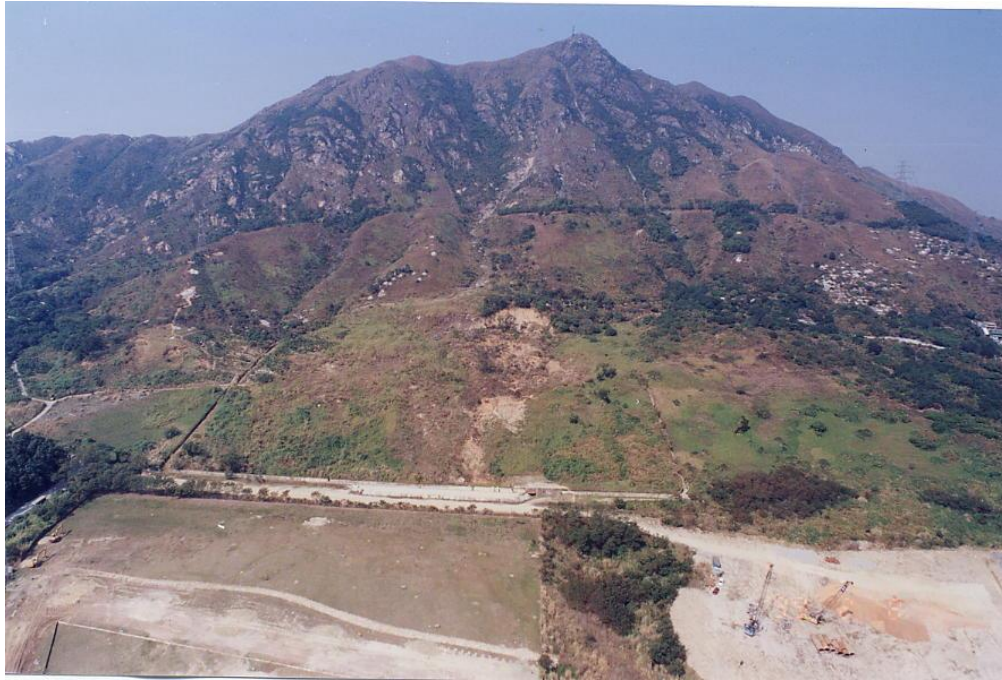
PLATE 2: Area 19 cut slope in the foreground and Tsing Shan massif above (before construction)
