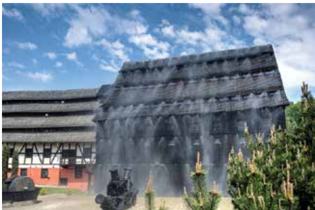
Photo 78. Water mist extinguishing system Archive of the Museum of Papermaking
