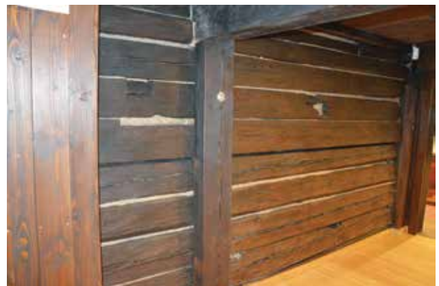
Photo 53. Log cabin structure of the oldest part of the drying house. Photo by A. Fortuna-Marek
