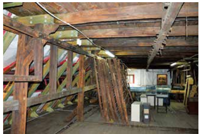
Photo 40. Paper mill attic, currently not used for any purposes. Photo by A. Fortuna-Marek
