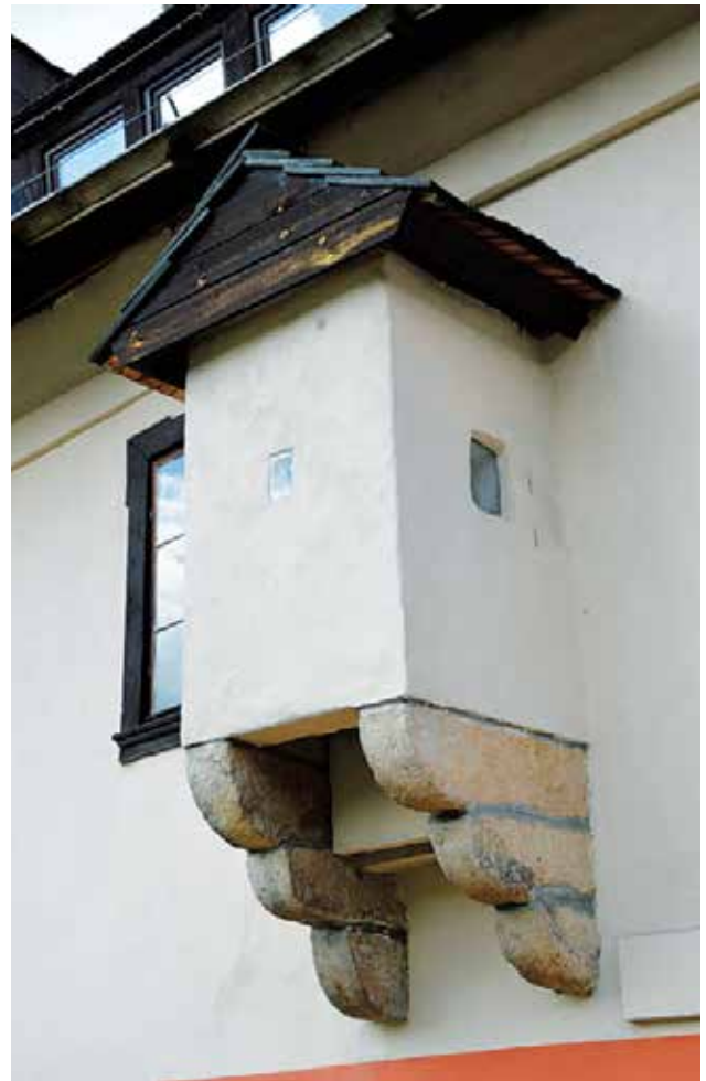
Photo 28. Bay window in the south-facing wall of the paper mill Photo by A. Fortuna-Marek
