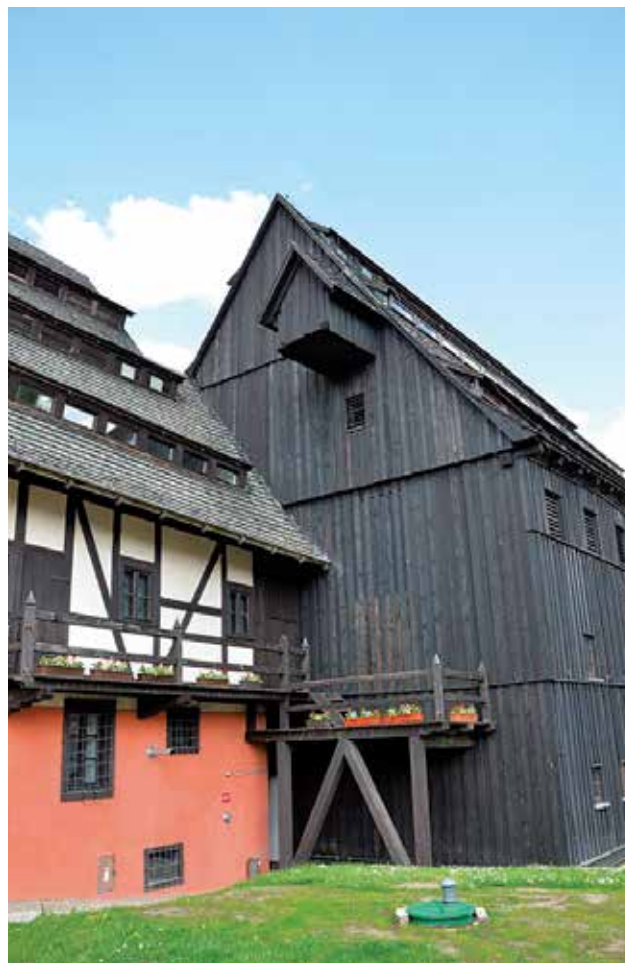
Photo 32. The mill and the drying house facing south-west Photo by A. Fortuna-Marek
