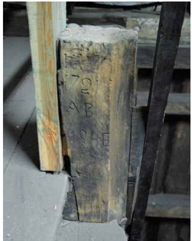
Photo 52. Staircase structural column in the paper mill building. Photo by A. Fortuna-Marek
