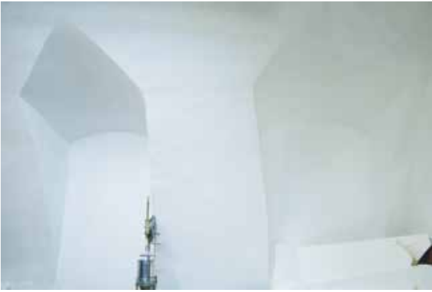
Photo 50. Paper mill building – barrel vault with lunettes in the lower ground floor. Photo by A. Fortuna-Marek
