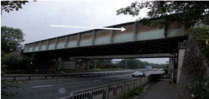
Fig 1.1 Typical U-Frame Railway Bridge showing atmospheric pollutant deposits arrowed.
