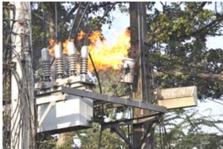
Figure 1. The transformer explosion caused in middle voltage (MV) [16].
