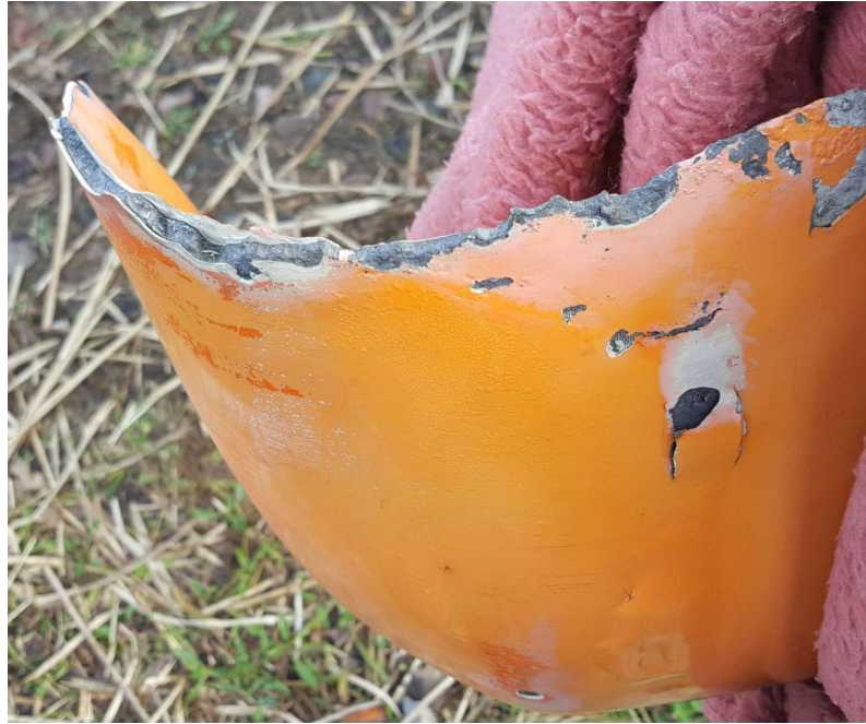
Figure 3.31: Cap type receptor (winglet) from wind turbine in winter lightning area after several years of operation. The lightning current degraded the trailing edge of the receptor.
