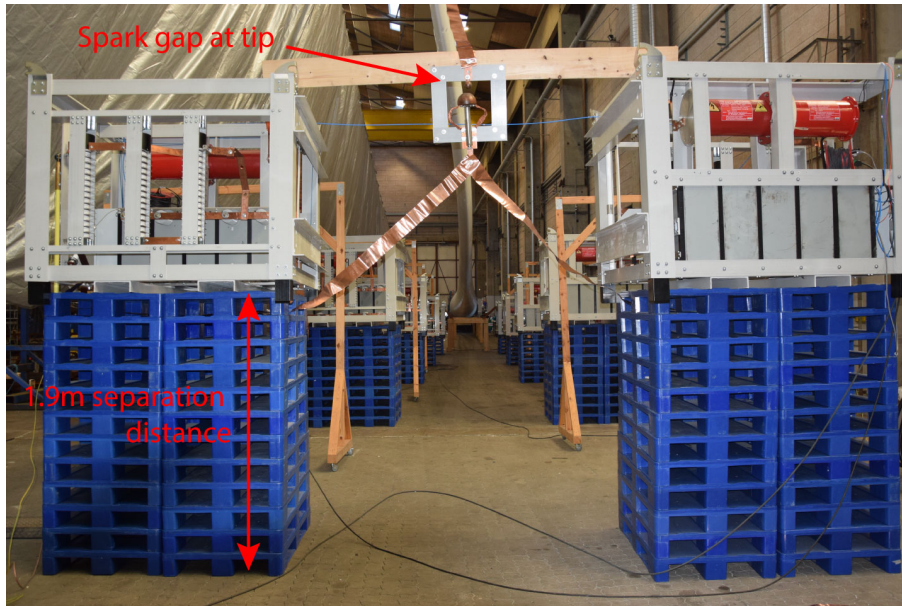
Figure D.1: The tip of the blade with spark gap and A-bank modules on isolating plastic pallets.
