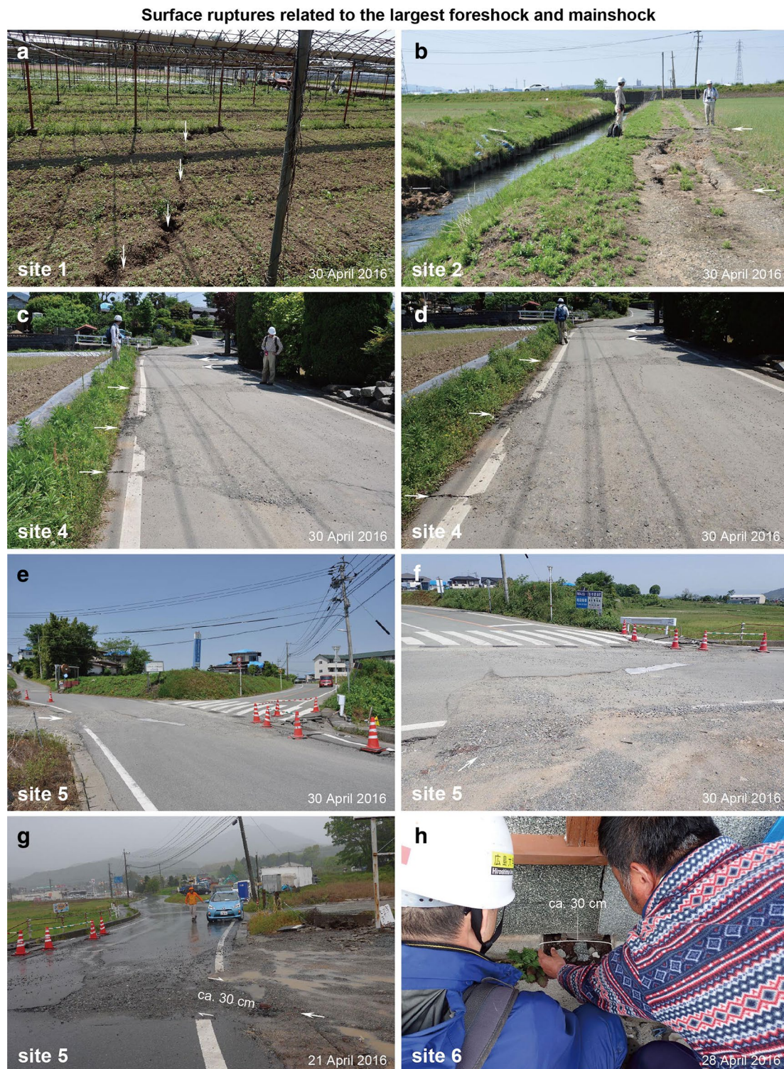
Fig. 4 Snapshots of surface ruptures related to the largest foreshock and mainshock at each site shown in Fig. 1c and/or Fig. 2. a Mole-track structures and open cracks, which first appeared associated with the largest foreshock and later enlarged due to the mainshock. b Two fault traces on an unpaved road, indicated by white arrows , between which a small depression appeared. Vertical offset of ca. 10 cm up on the north was identified across the two fault traces. c, d Five rupture traces with right-lateral offset of a paved road. Total amount of offset was 13–14 cm. e–g A fault trace on a paved road with right-lateral offset of ca. 30 cm. h An open crack of a concrete block, whose width was ca. 5 cm after the largest foreshock and ca. 30 cm after the mainshock
