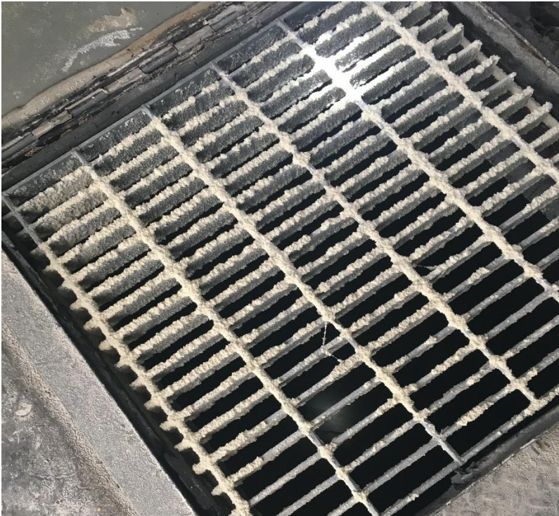
Figure A-1. Receiving ingredients pit grating
