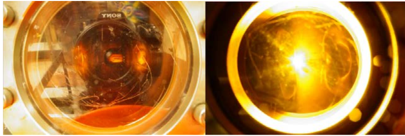
Figure 4-3: Photograph of the oil gap switch pre-fire (left) and during operation (right).
