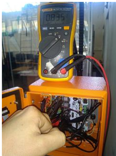
Figure 5.4: Adjusting Motor Trim-pot Current to Acceptable Level
