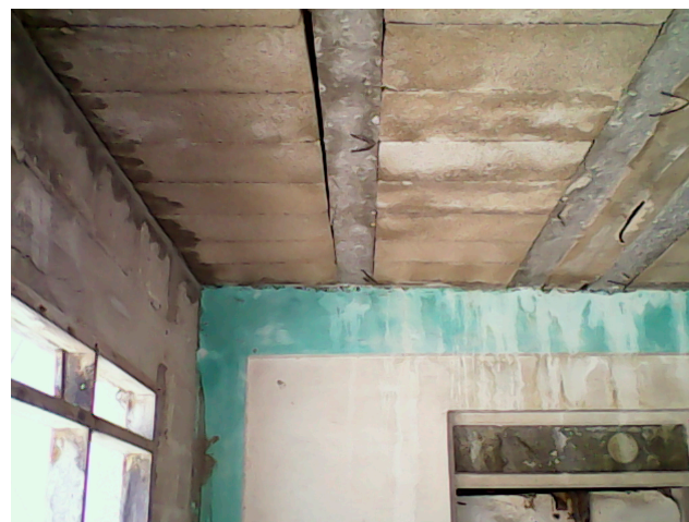
Figure 5. Interior of house showing moisture damage (Photo: J. Biles).
