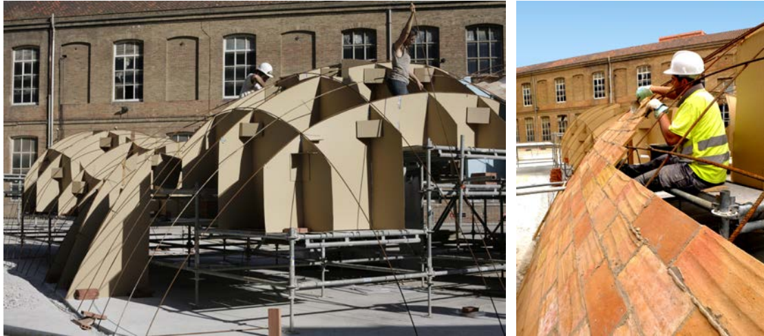
Figure 5: a) Construction of the falsework with cardboard sections and rebars; and b) building the vault on the falsework. © Manuel de Lózar and Paula López Barba.
