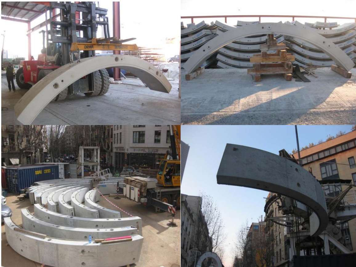
Figure 7. (a) Transport after mould release; (b) provisional support under storage; (c) support configuration in the work zone; and (d) lifting operation for the placement of the ring.
