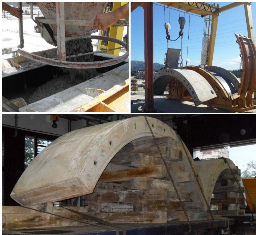
Fig. 12. (a), Concrete pouring (b), demoulding operation and (c) transport of the segments.
