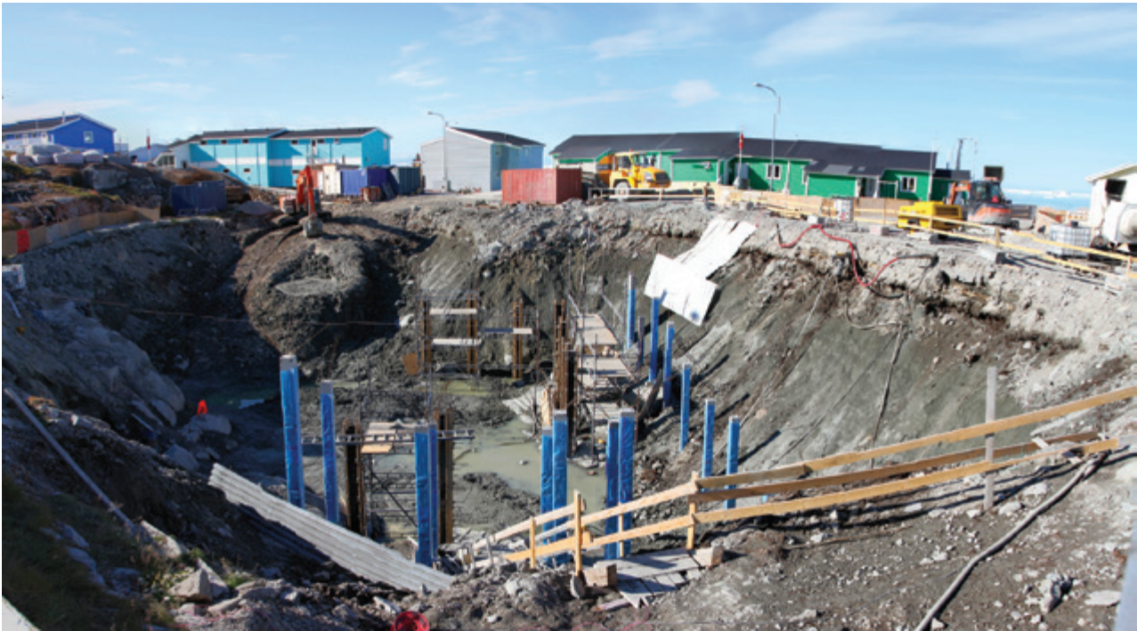
Figure 10.27 Excavation and in situ casting of piles for the new district court house in Ilulissat, August 2015. The photo illustrates the current practice of excavating to bedrock for in situ casting of piles anchored in the bedrock, followed by backfilling (photo by Thomas Ingeman-Nielsen).
