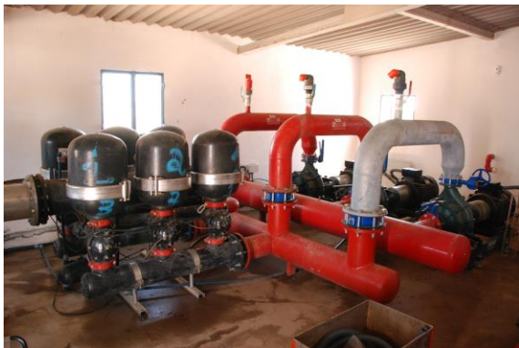
Figure 4: Set of pumps and filter bench
