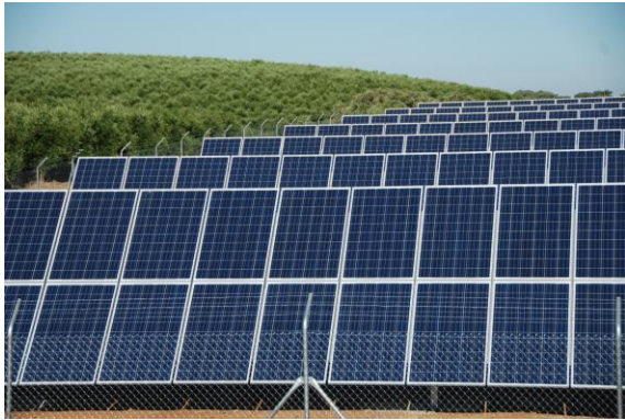
Figure 3: PV system generator
