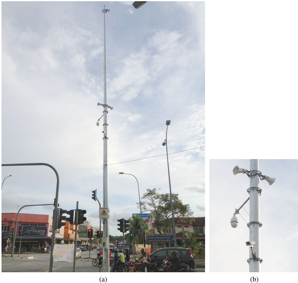
Figure 1.1: Surveillance cameras installed at traffic light junction in Malaysia: (a) surveillance cameras installed at the middle section of the pole; (b) close up view of the surveillance cameras.
