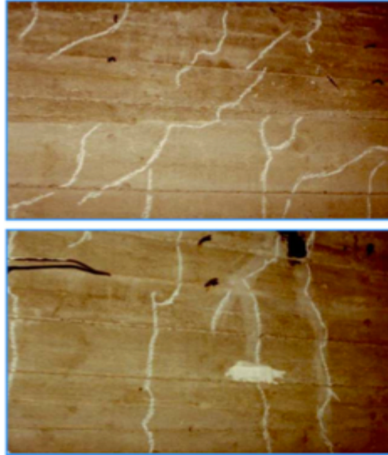
Figure 6. 1- Cracks noted on two beams (Shash et al. 2005).
