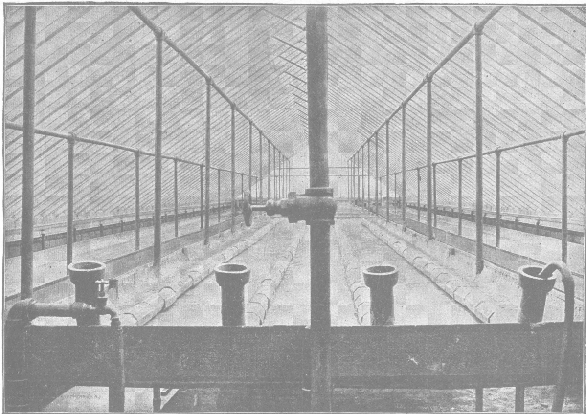
FIG. III.—INTERIOR OF GREENHOUSE, SHOWING BENCHES WITH BOTTOMS CEMENTED, AND IRRIGATING TILE LAID.
