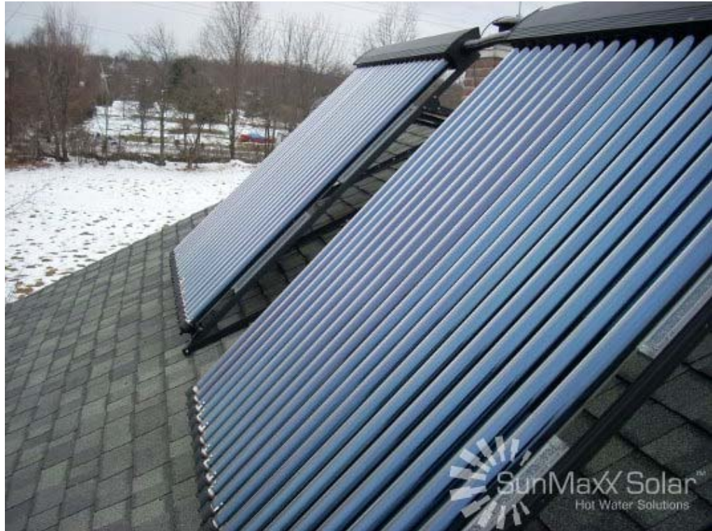
Figure 12: Evacuated solar tubes
