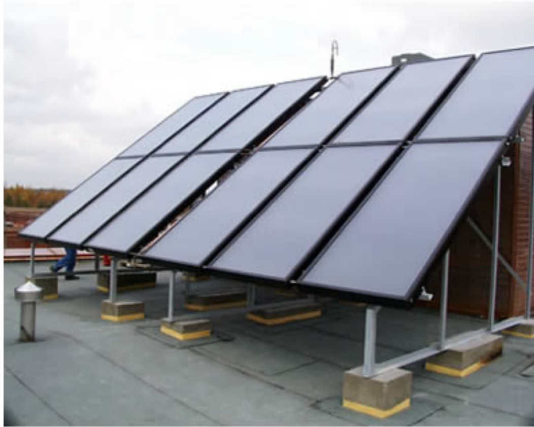
Figure 11: Solar Flat Plate Collectors
