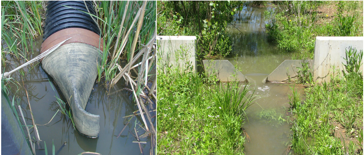
Figure 2. Inflow and outflow control structures in the created oxbow wetland. The Red Field Tideflex™ check valve, left, opens via water pressure when the river elevation is higher than the wetland and then recloses when the river elevation is lower than the wetland water level, and water pressure is removed. Water then flows back to the Olenyangy River through an outflow control weir, right.
