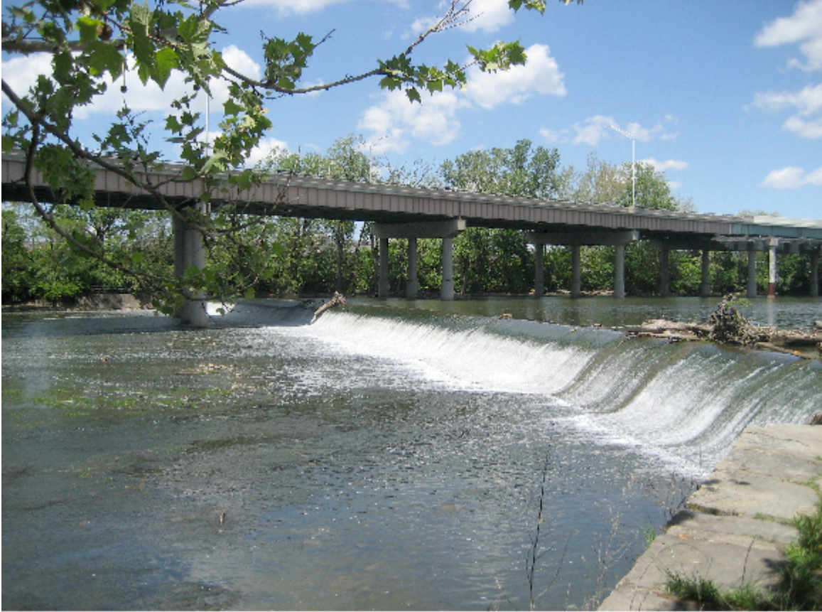
Figure 2. Fifth Avenue Dam and a portion of the upstream created reservoir. (photograph by Alexandra Naegele)
