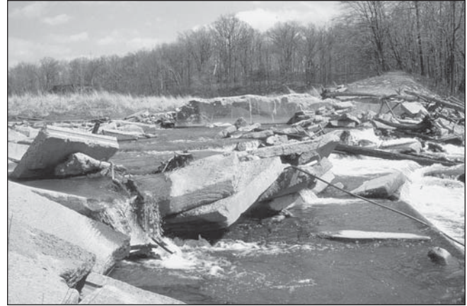
FIGURE 8-6.—View of the former dam site after removal of the spillway and conversion of the former reservoir to riparian wetlands. Photo by J. Evans.
