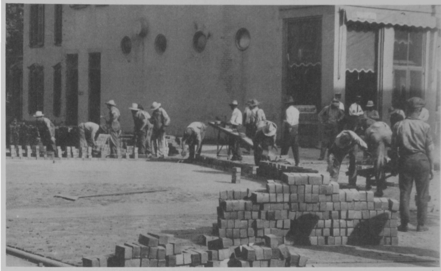
The popularity of the automobile increased the pressure on local government for paved streets. After much controversy, in 1925 the village council approved paving Main Street with brick. Workers are shown assembling their bricks at the corner of Main and Central. Courtesy Camden Archives.
