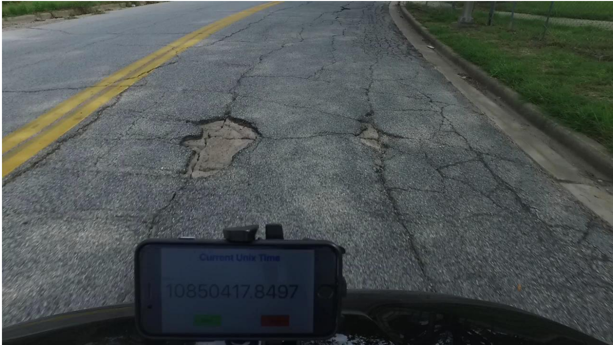
Figure 2. A frame shot with the Osmo showing a pothole
