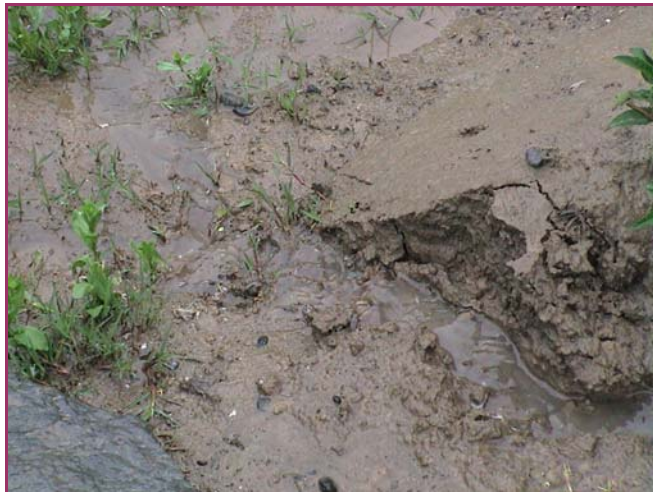
Figure 14. Water runoff and erosion effects during heavy rain at the Kharga site
