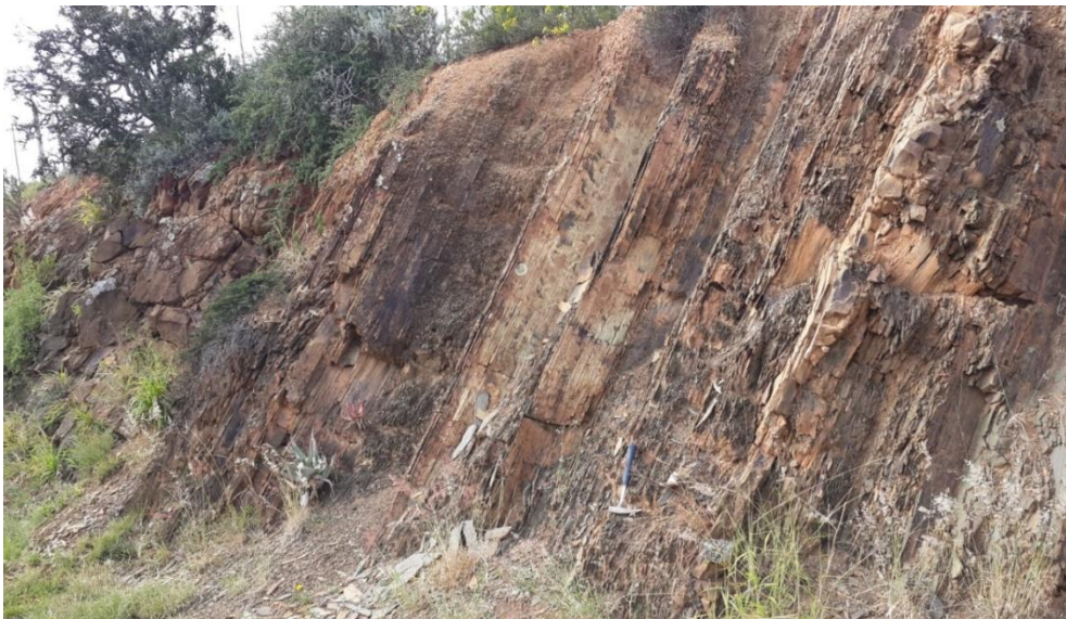
Figure 3.9: Photograph showing the near vertical dark-grey shale of the Whitehill Formation along National road N2 between Grahamstown and Peddie.
