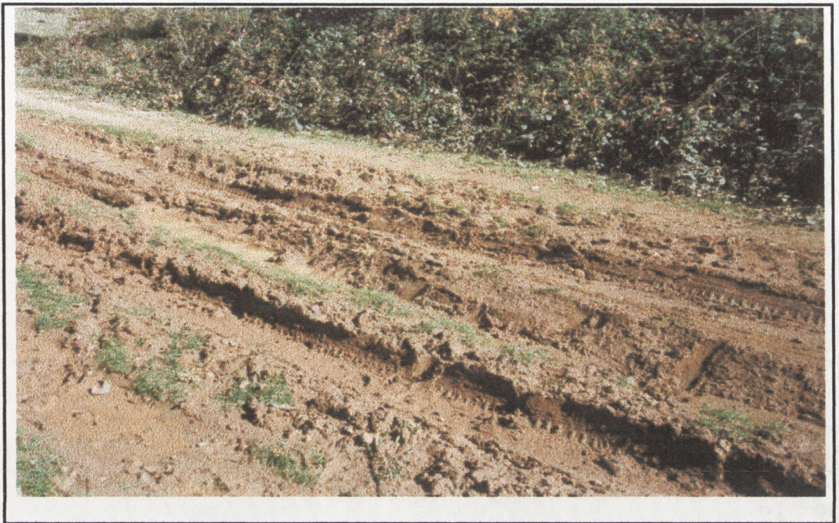
Figure 2.2 Example of Rutting on a Forest Road (Bago State Forest, 19/5/98)
