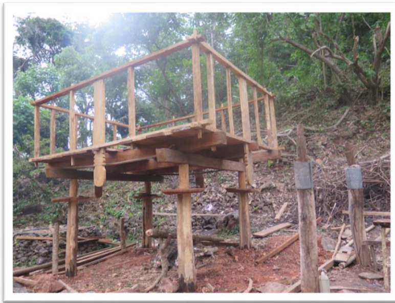
Figure 1.14: Oma falu structure installed at Bubuha, Larisula, Baguia Sub-district, 16 August 2014. Note the original sa'a are situated to the right, beside the newly constructed oma falu .
