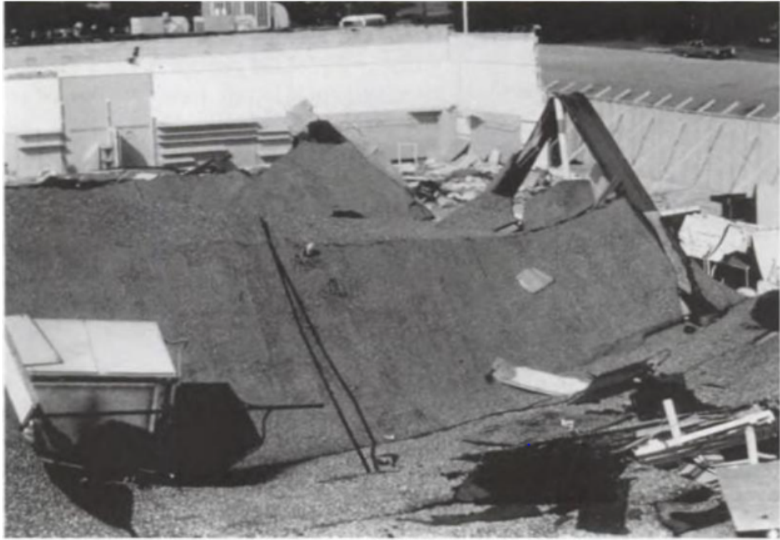
Figure 2.4 : Collapse of a Department Store in Bolivar [6].
