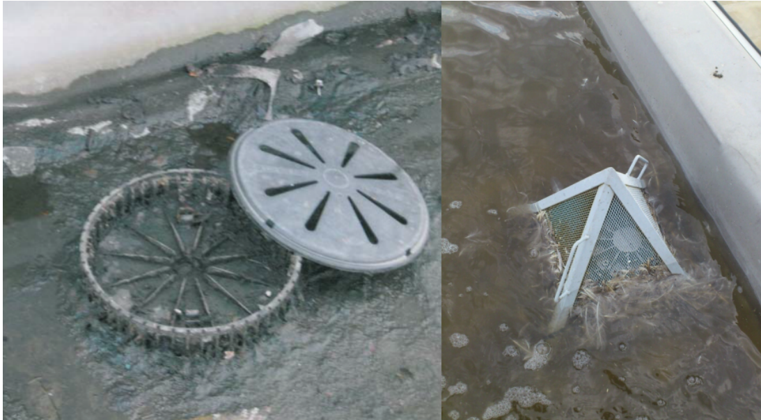
Figure 3.1 : Blocked Primary Drainage.
