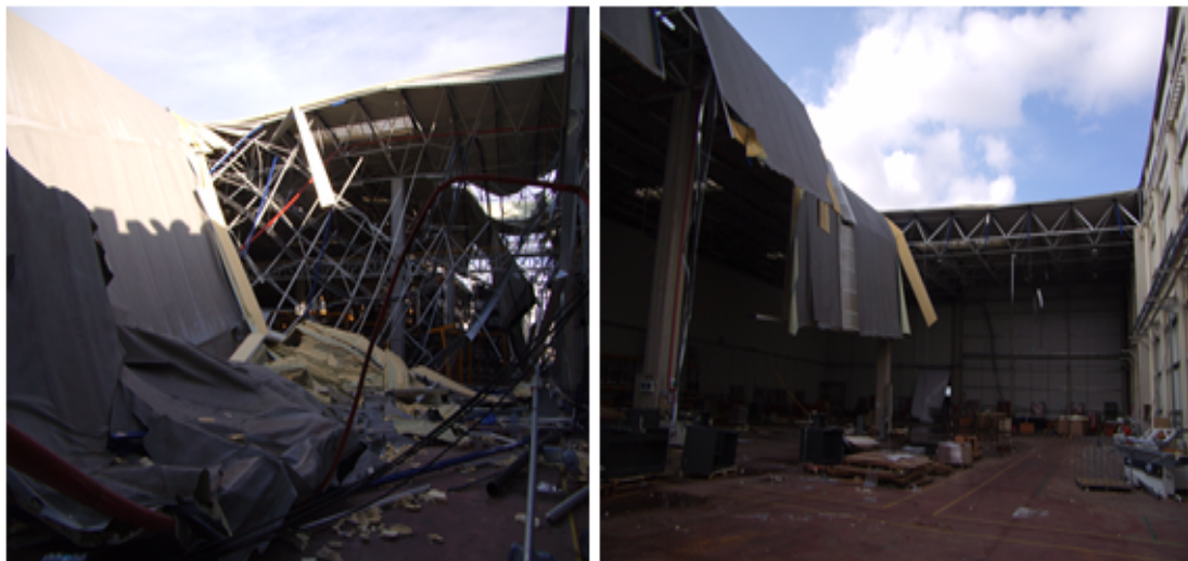
Figure 2.5 : Collapse of a Factory in Istanbul [7].
