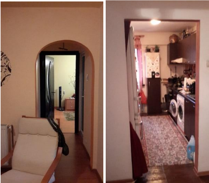
Figure 4.15: Doors removal in the case of F8 (left) and for F9 (right).
