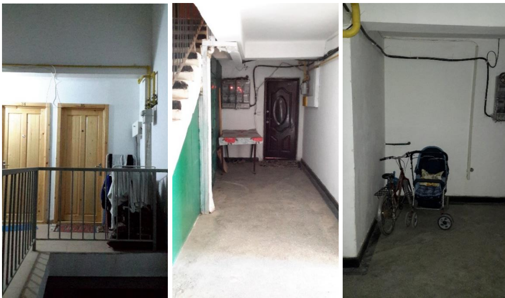
Figure 4.21 Door fronts used as storage in block 'N'.
