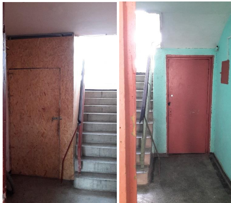
Figure 4.24: Storage spaces built under the stairs in both segments of block 'D'.
