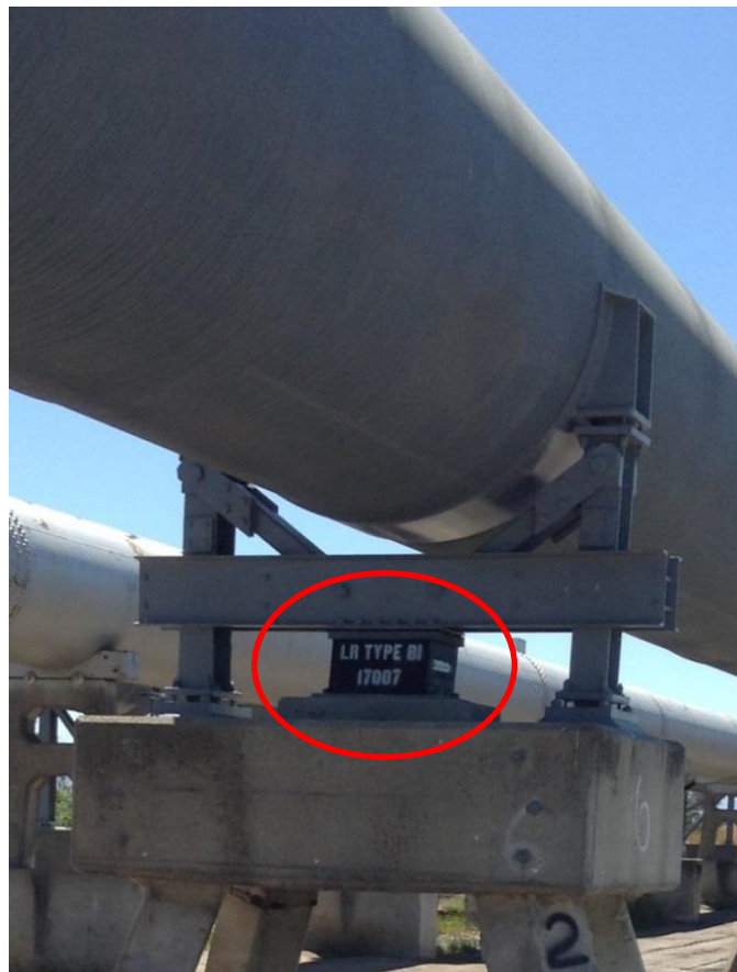
Figure 7. Aqueduct No. 3 seismic upgrade, Sacramento-San Joaquin Delta, California. June, 2017. Base isolator on Aqueduct No. 3 (2000).
