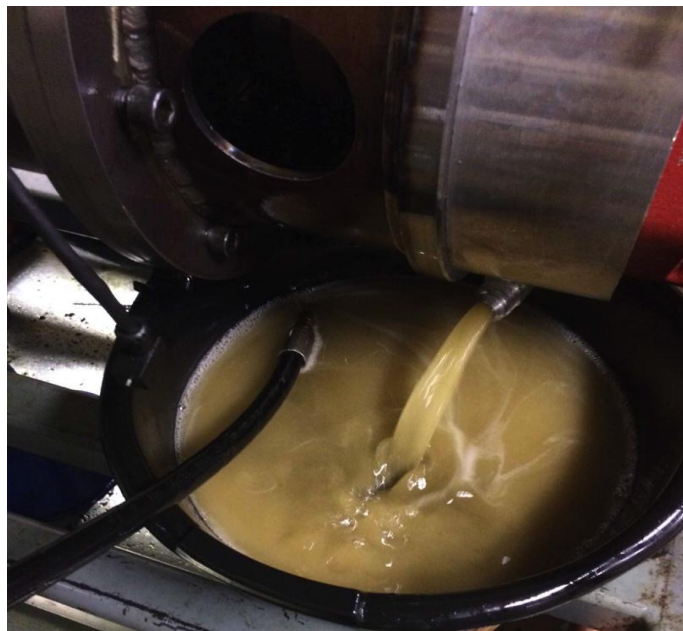
Figure 4.15. Case drain for lubrication flow, highly aerated.
