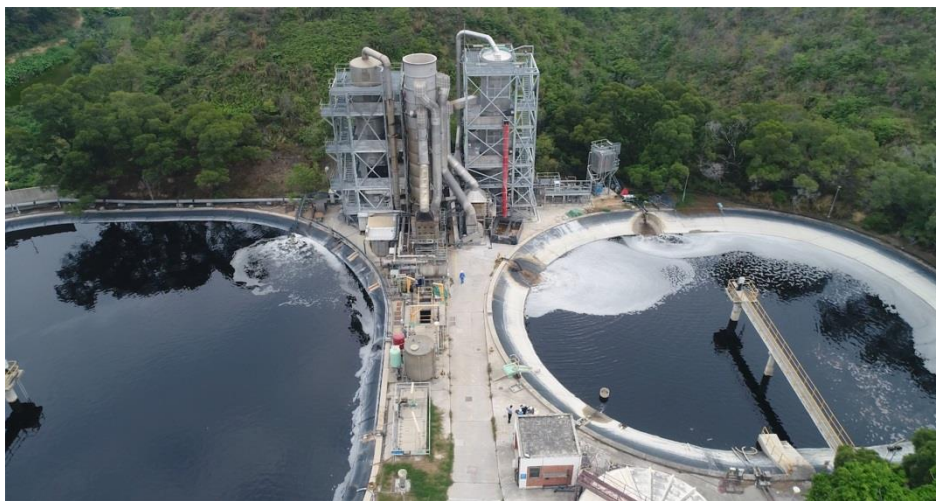
Figure 2.2: Full scale plant for treatment of landfill leachate by ammonia stripping (Organics, 2018)
