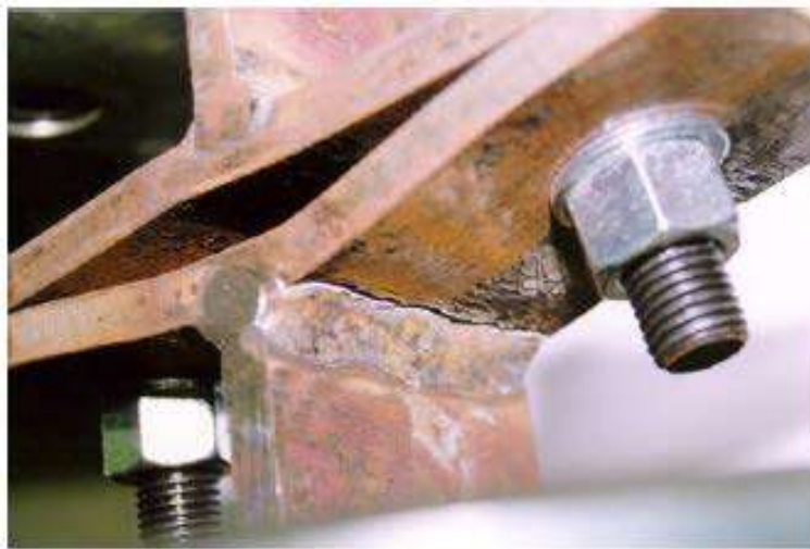
Figure 2.2: Failure mode of specimen under cyclic tests [8]
