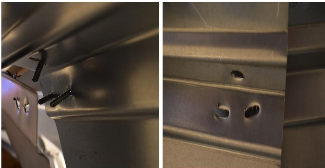
Figure 35 Bearing around screw holes and detachment of sheets
