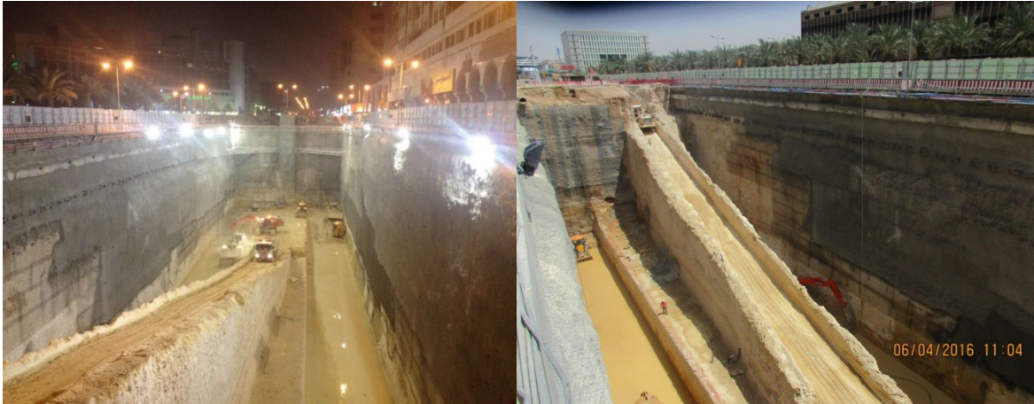
Figure 16. Excavation of one station with this solution. Ramp over the tunnel crown.
